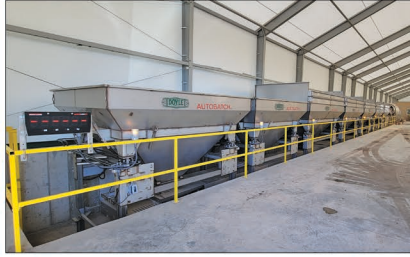
Multi-hopper automated blend system features two swing hoppers, each with a 9-ton capacity.
